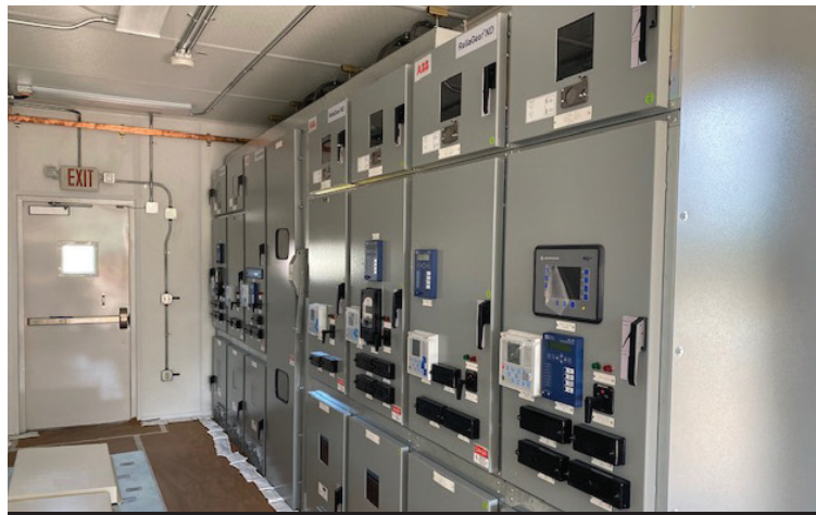
PEARL microgrid's Power Distribution Center; the control room for utility and cyber security systems
