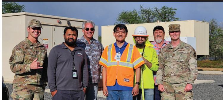
Members of the PEARL microgrid team from the 154th Civil Engineer Squadron, Burns and McDonnell, and Hitachi
